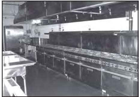
Ovens and Stoves, Kitchen
